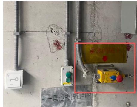
辐照室急停及拉线开关
